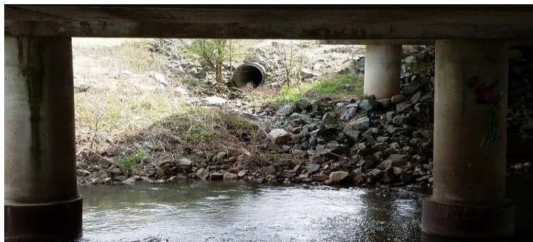
Fig. 1 – Photo showing sewage pipe that empties directly into Salem Creek. April 02, 2015. Photo: Ilyina O. L.
